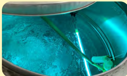
Sterilization lights on RO water tanks installed by local engineers
